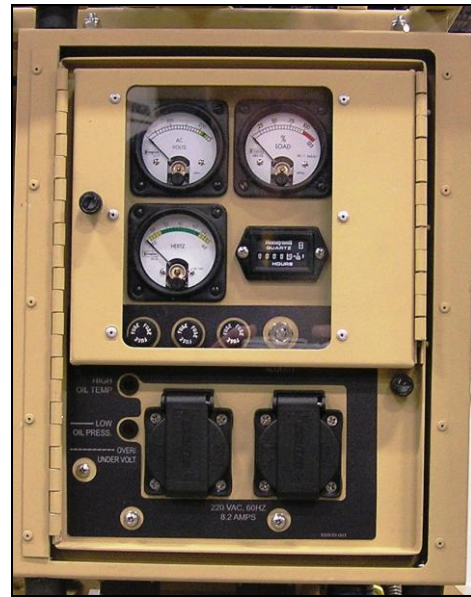
Front Control Panel
